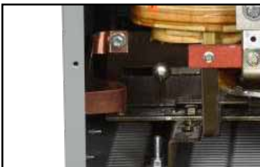
Factory installed main grounding lugs
